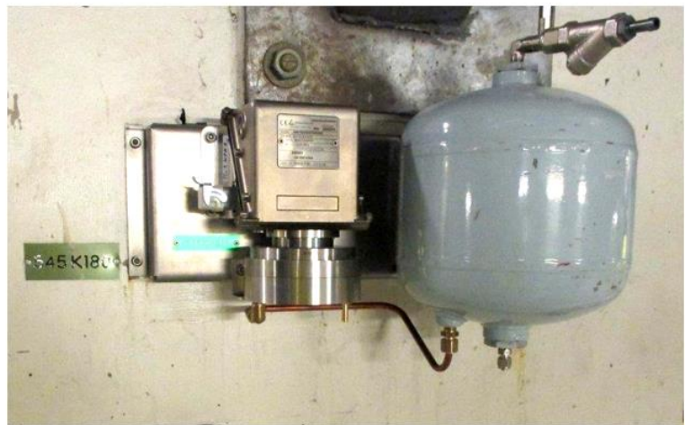
DP Switch Measuring HELB in Containment
