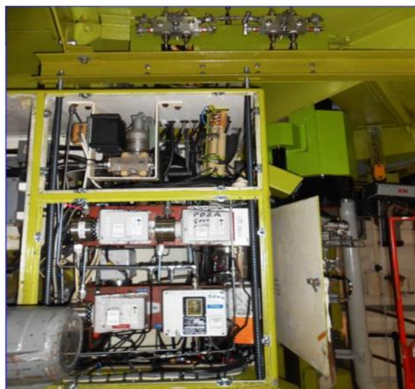
Switches in Fuel Charge Unit
