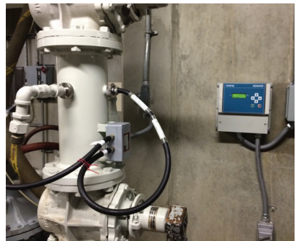
Mobrey MSM400 controller and sludge sensor installation
