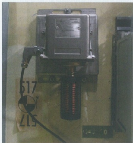
Fast Response Air Temperature Switch installed inside a NPP.
