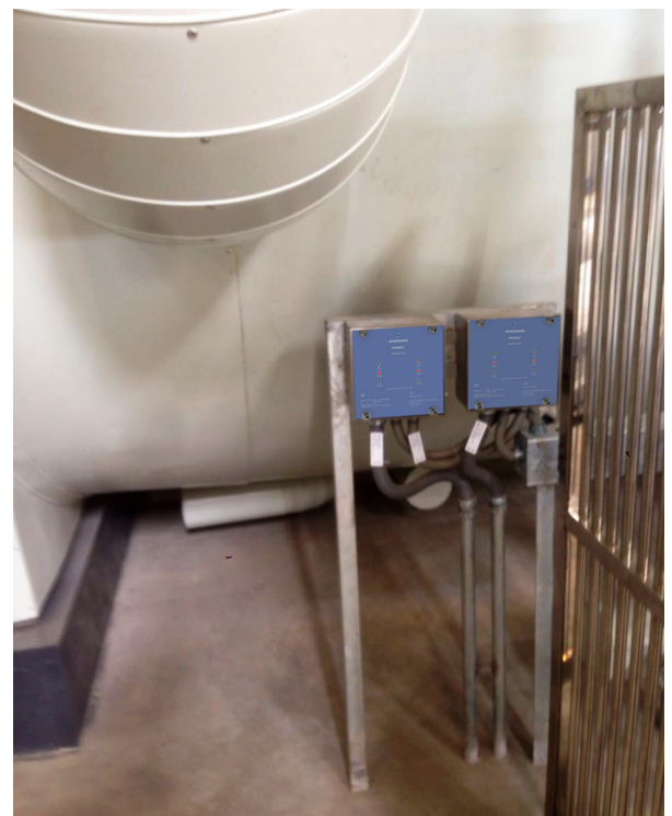
Mobrey Hydratect's are installed on the steam lines.
