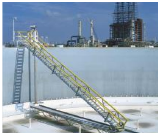
Potentially dangerous spillage is prevented using the Delta Mobrey vertical switch
